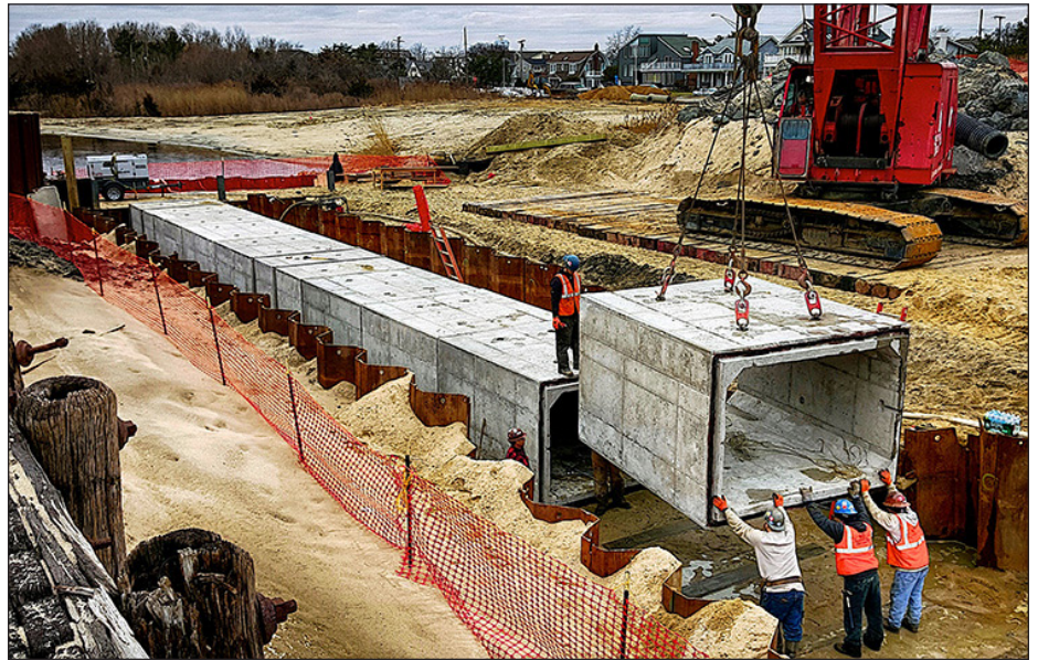
The 600-foot passage at Wreck Pond will make it easier for migratory fish to move into and out of the pond, while also improving water quality and reducing local flooding.
